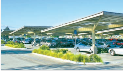
A parking lot in San Diego is shaded by solar panels that provide energy for buildings on the site.
